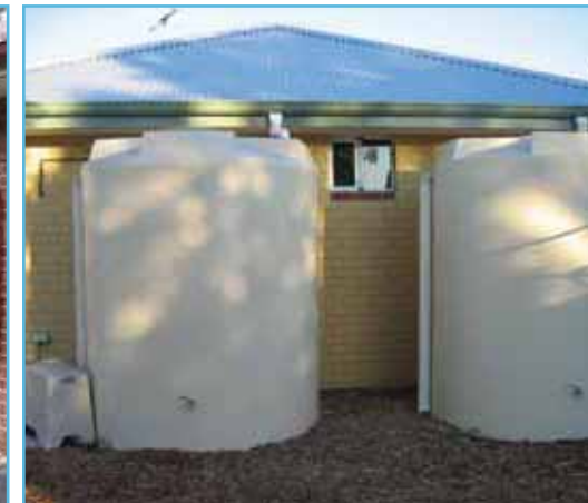
Poly domestic rainwater tanks
