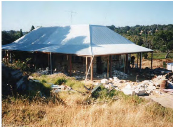
Image of conservation works 2013. Courtesy Heritage Report for Thorn Hill (fmr) Lot 772 (3) Coley Road Yallingup WA.
