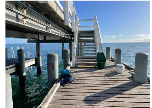
Photo 51: View of swim platform 5B, east side of Jetty Section 5, Busselton Jetty. H+H Architects, 2022.
