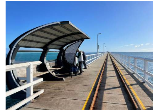
Photo 53: View of curved shelter used by fishermen, Jetty Section 5, Busselton Jetty. H+H Architects, 2022.
