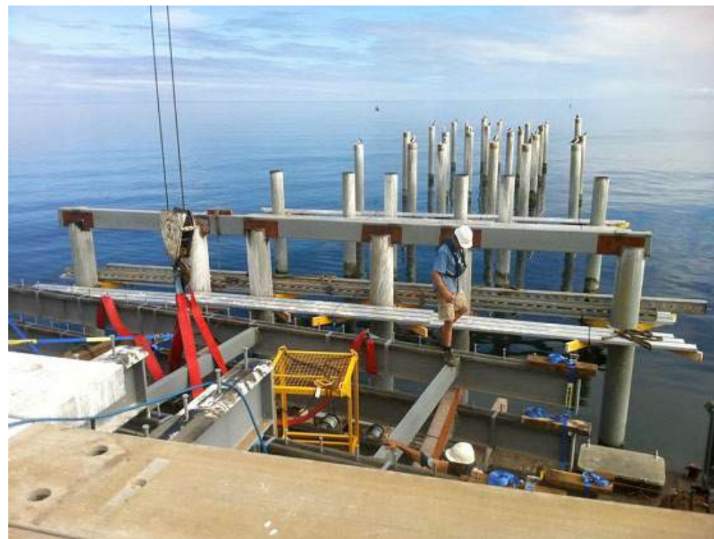
Image 38: Replacement of piles and headstocks underway at Busselton Jetty during 2013. SMC Marine.
