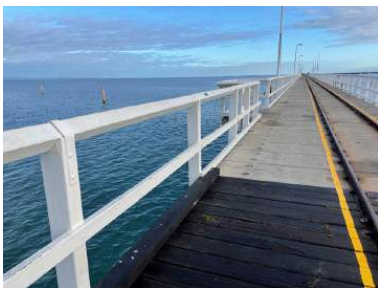
Photo 1: View of transition between timber/concrete decking and kerb-rail and balustrade details. H+H Architects, 2022.
