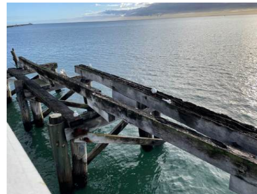
Photo 41: View of Interpretive Node #3 showing remaining timber jetty bents and stringer/rail beams affixed to half-caps. H+H Architects, 2022.
