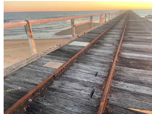
Photo 74: Detail view of remaining train tracks to timber deck, and remnant timber balustrade, Carnarvon One Mile Jetty. H+H Architects, 2022.
