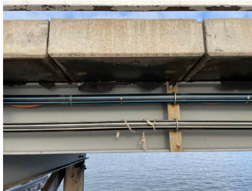
Photo 36: Detail view of steel stringer beam and concrete deck, Section 2. H+H Architects, 2022.
