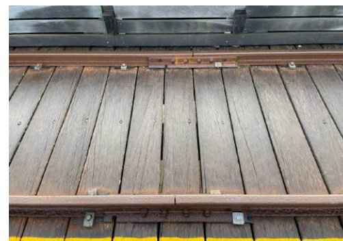
Photo 19: Detail view of timber deck and rail track to Jetty Section 1- West. H+H Architects, 2022.
