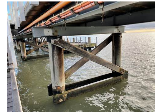
Photo 22: Detail view of jetty bent with timber piles and steel superstructure to Section 2. H+H Architects, 2022.
