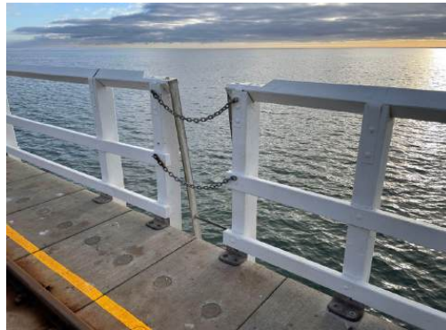
Photo 24: Detail view of typical safety ladder & chain gate, Section, Busselton Jetty. H+H Architects, 2022.
