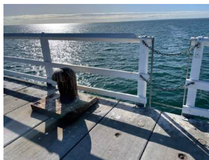
Photo 64: View of ladder and salvaged bollard at the Jetty Head, Busselton Jetty. H+H Architects, 2022.
