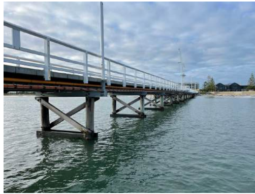
Photo 26: View of typical jetty bent detail with timber piles and steel superstructure, Section 2, Busselton Jetty. H+H Architects, 2022.
