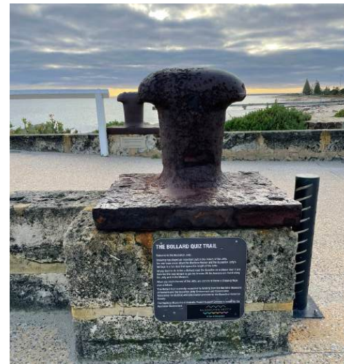
Photo 3: View of salvaged bollard which forms part of the Bollard Trail across Busselton Jetty. H+H Architects, 2022.
