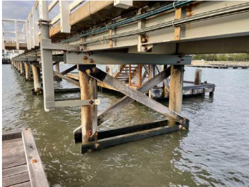
Photo 35: Detail view of Jetty bent detail to Jetty Section 2 showing outrigger support for light poles. H+H Architects, 2022.
