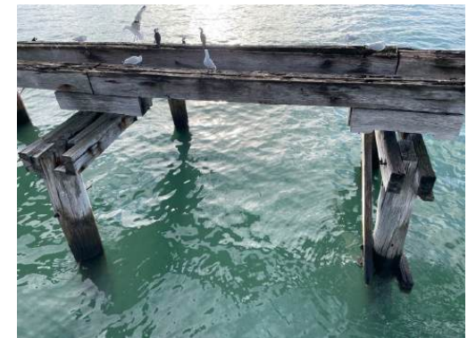
Photo 42: View of Interpretive Node #2 showing remaining timber jetty bents and stringer/rail beams affixed to half-caps. H+H Architects, 2022.
