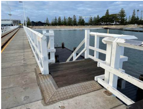
Photo 25: Detail view of upper landing to Platform 2B, Section 2, Busselton Jetty. H+H Architects, 2022.
