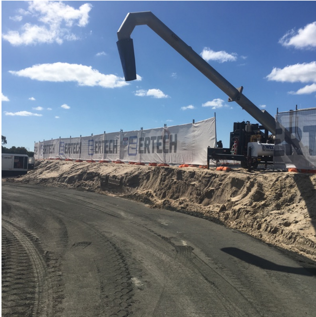
Turkeys nest dam access & pump
